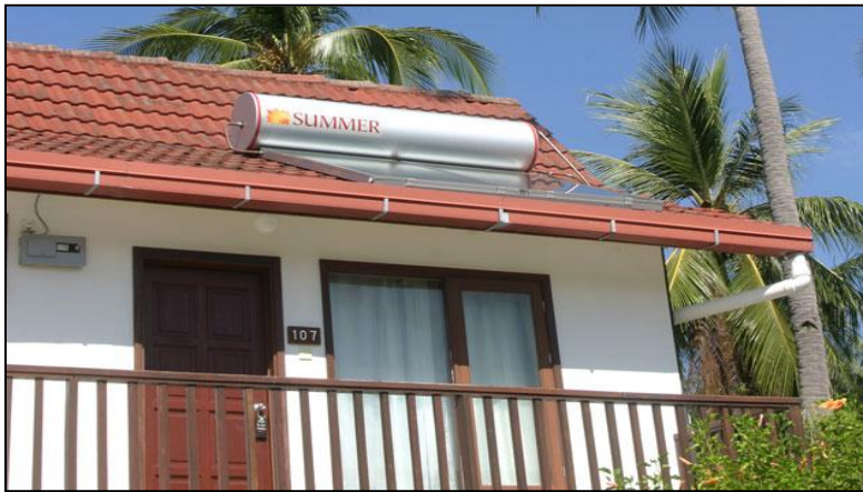
FIGURE 2 – SOLAR PANELS AT FRANGIPANI RESORT
