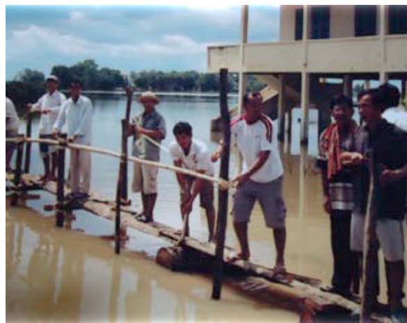
Impact of Flooding: A resourceful community builds a temporary bridge to keep their school open during a flood on the Mekong River.
