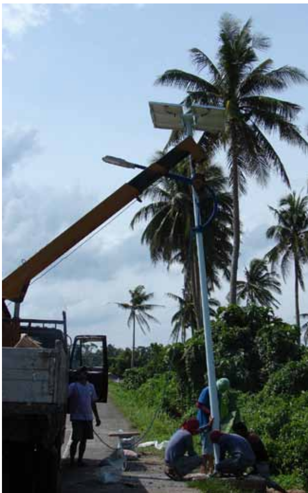
Installation of a solar-powered street light along Diversion Road in Sorsogon City, Philippines.
