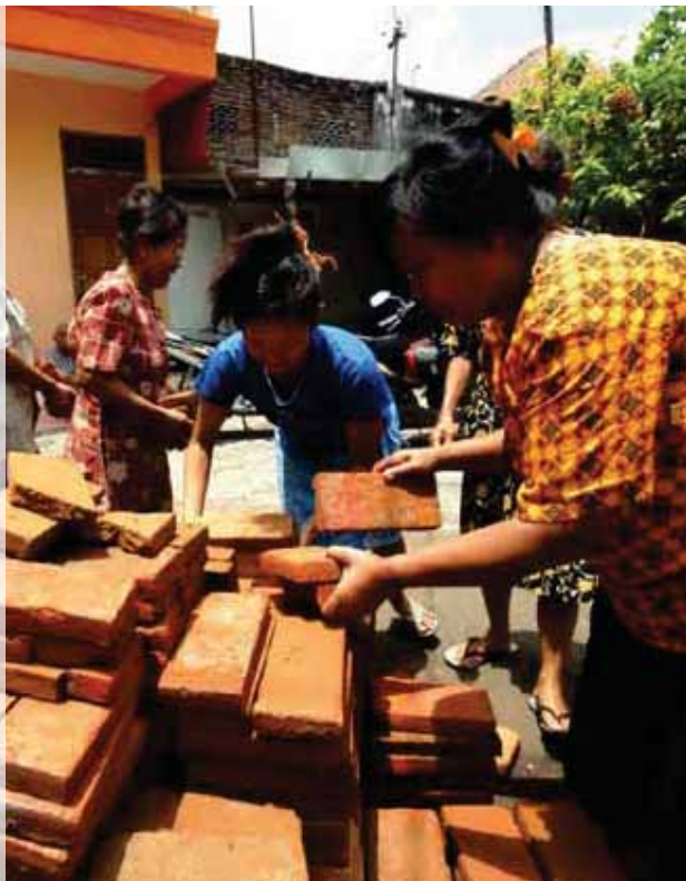
Women in Solo, Indonesia carry materials for upgrading their houses ©UN-Habitat/Ruth McLeod.
