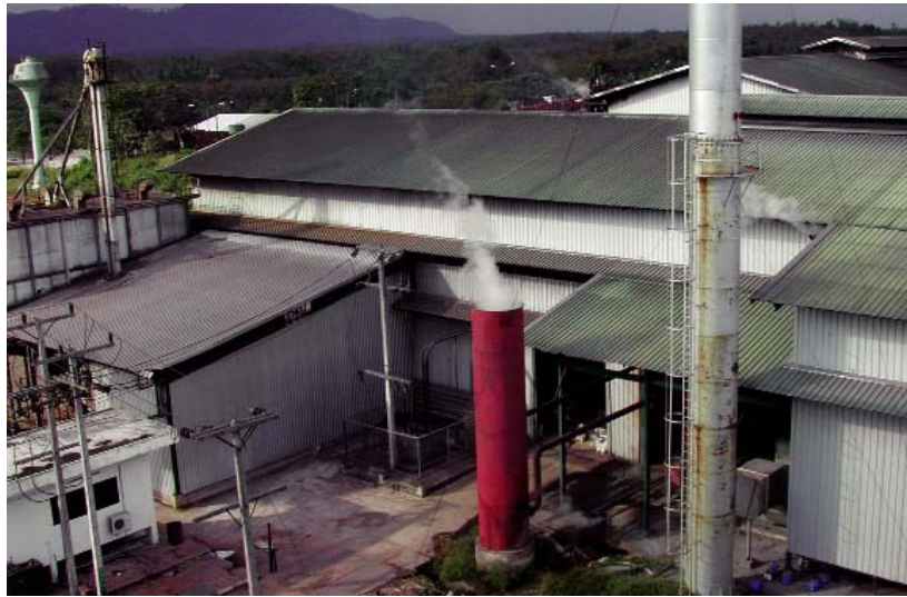
A 1 MW Rice Husk Biogas Generation Plant in Thailand.
