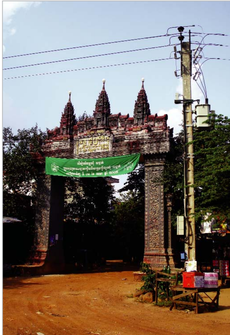
A Transmission Line in Cambodia. Photo courtesy of International Rivers.
