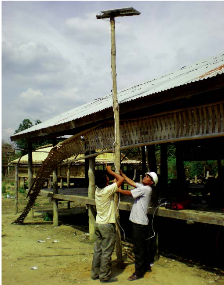
Solar Panel Installed for a Remote Literacy Class in Rattanakiri Province. Photo courtesy of Clean Energy Group.
