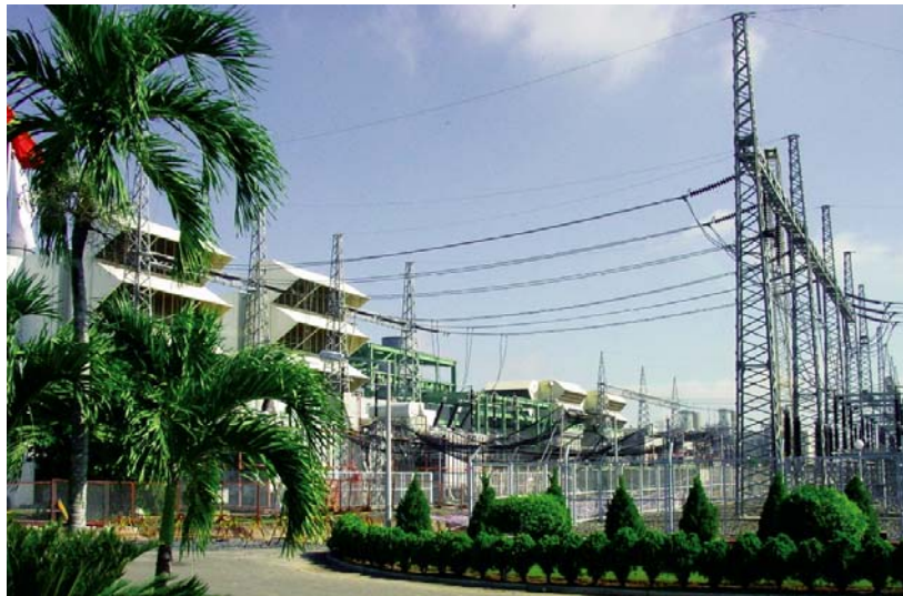
The Phu My Complex, a Combined-Cycle Gas Turbine Power Plant in Southern Vietnam.
