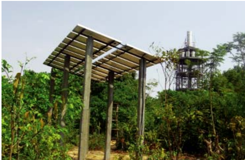
Solar Panels in Kampot Province Used to Run a Solar Pump, which Fills the Water Tower in the Background. Photo courtesy of Clean Energy Group.
