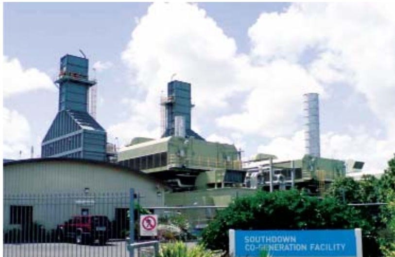
Southdown Cogeneration Facility in New Zealand.
